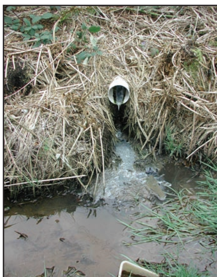
Figure 2: Direct Discharge from a Straight Pipe
